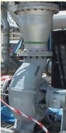
Below: Cooling water pump for primary turbine at a power plant in the Middle East.
