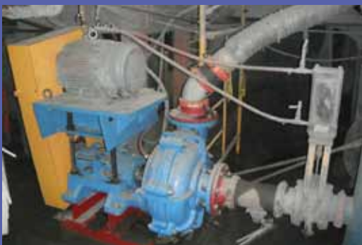
Primary Cyclone Feed Pump in a Primary Metals Mill
